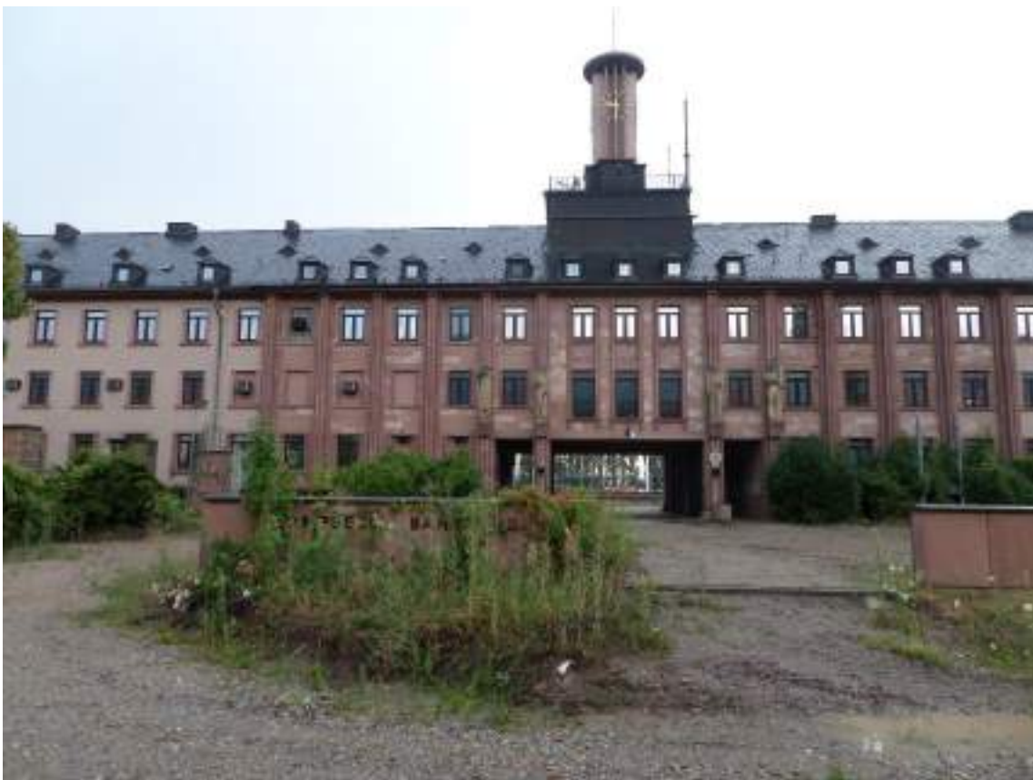
State of abandonment of the Campbell barracks in Heidelberg (Germany). Source: photo by Federico Camerin (2018).
