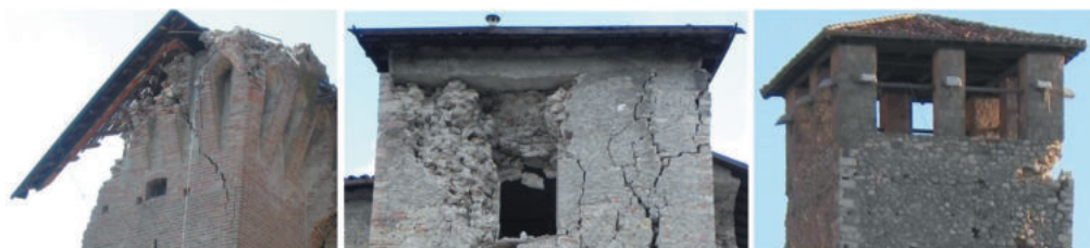
Figure 6. Shear collapse of the roof structures in San Felice sul Panaro Castle (Emilia); Tower of Norcia curtain wall (Central Italy); Kruja Castle (Albania).
