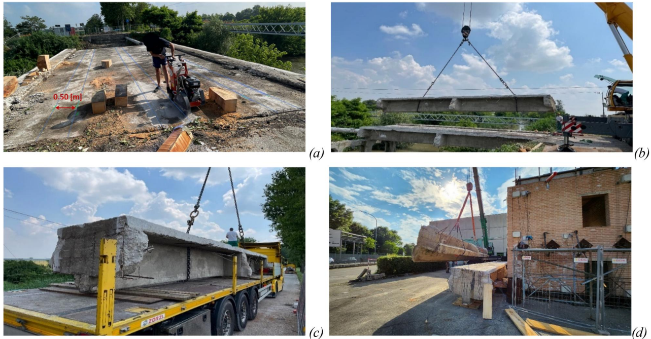
Figure 9. Main phases of the demolition process: (a) cutting of the slab and demolition of the transverse beams; (b) lifting of the girders; (c) loading the beams onto the truck bed; (d) positioning of the girders at the CIRI-EC structural testing laboratory of the University of Bologna.
