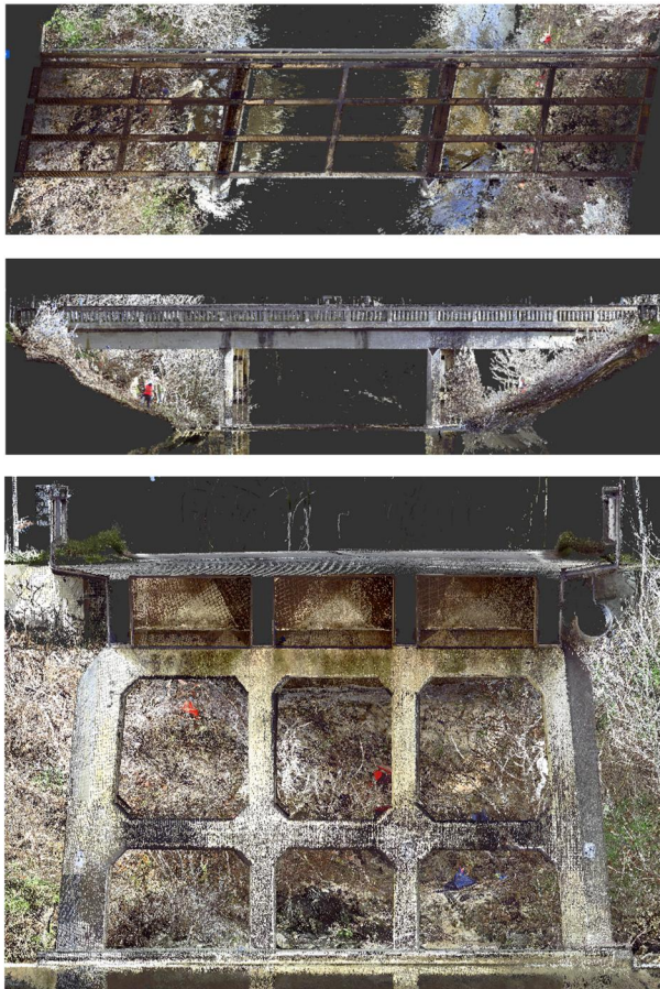
Figure 3. (a) Top view; (b) lateral view; (c) cross-section of the Fratta bridge.
