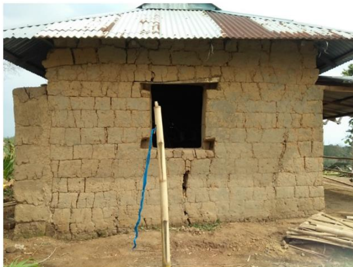
Figure 2.3: Cob building with extended shrinkage crack pattern [53]
