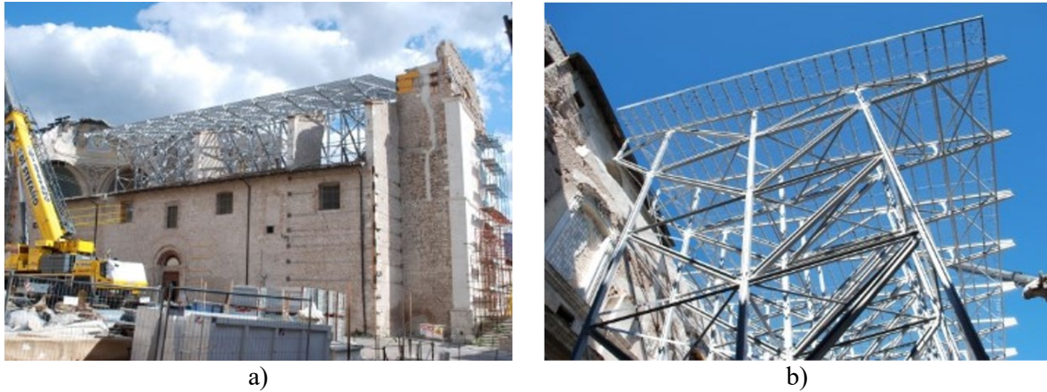
Figure 1: View of the fibre-polymer composite structure that protects the earthquake damaged Santa Maria Paganica church: a) general view of the partially collapsed church with top of composite structure; b) view of the spatial frame structure looking up at its roof
