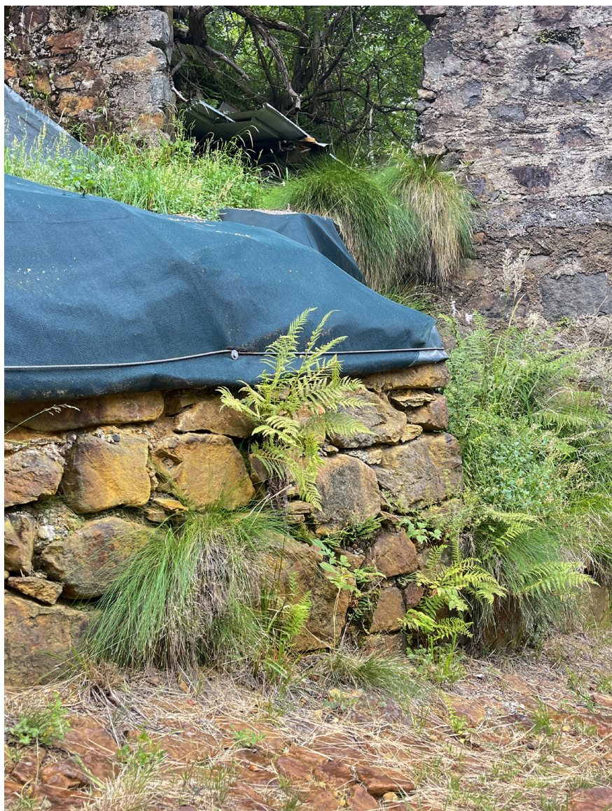
fig.10.30 Nickel deposit secured for safety reasons; the surface discoloration clearly reveals the effects of runoff and leaching. Campello Monti ( photograph by the author, 2023 ).
