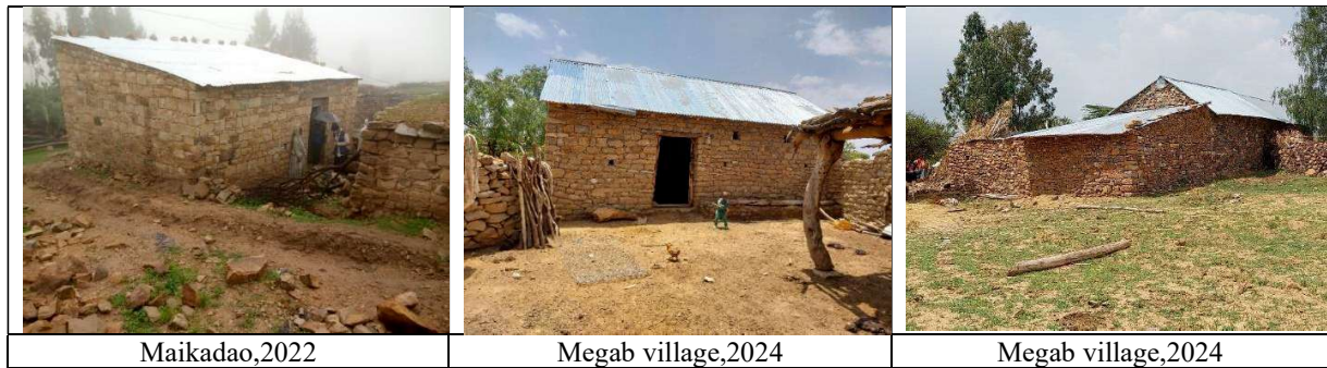
Figure 160: Hidmo housing reconstruction: flat roof replacement shade and open gable CGI roof (Source: author 2022 and 2024)
