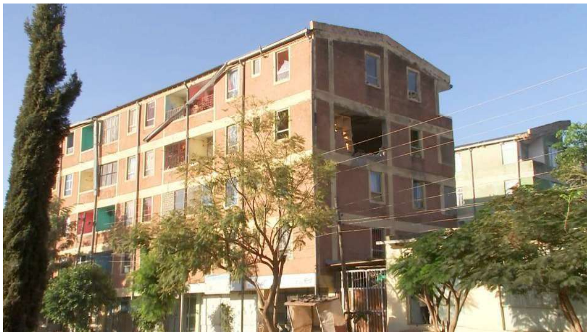
Figure 153: Damaged to wall of condominium building in Shire, Tigray, 2020 252
