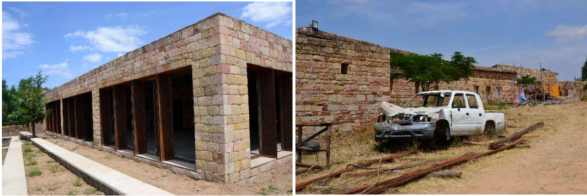
Figure 190: Burnt and damaged of Gheralta lodge after the war 2020-2022: (Source: Patassini D., 2024)
