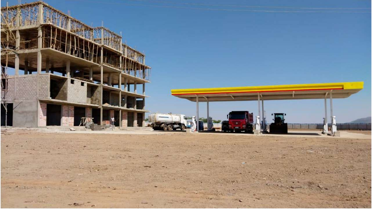
Figure 130: Fuel station under development at the junction of the asphalt road leading to the camp (Source: author 2025)
