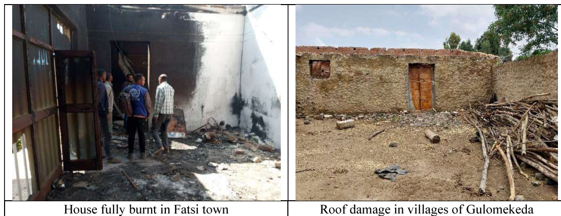
Figure 161: War-Inflicted Housing Damage, Gulomekeda (Source: authore,2024)
