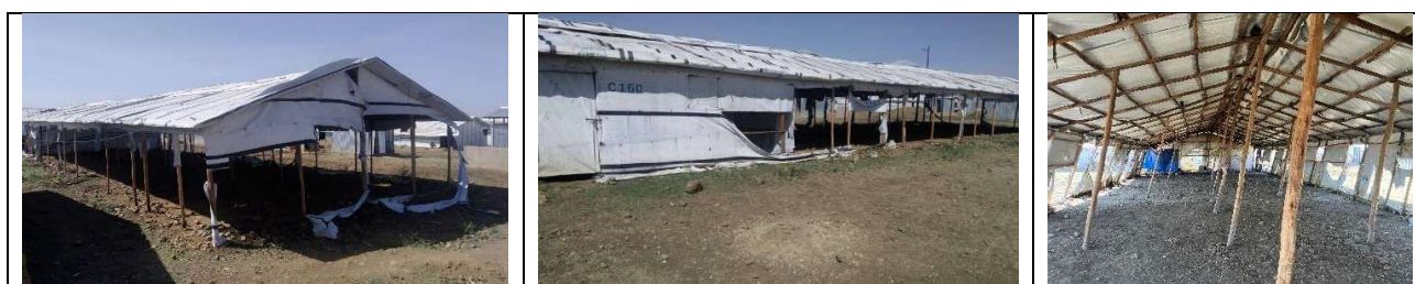
Figure 86: Communal shelter non-operational due to looting and vandalism (Source: author 2023)
