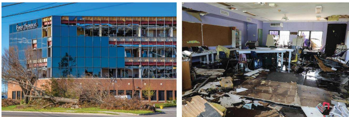
Figure 6. Flying debris damages on a building façade and view of a floorplan damaged by the combined action of rain and wind.
