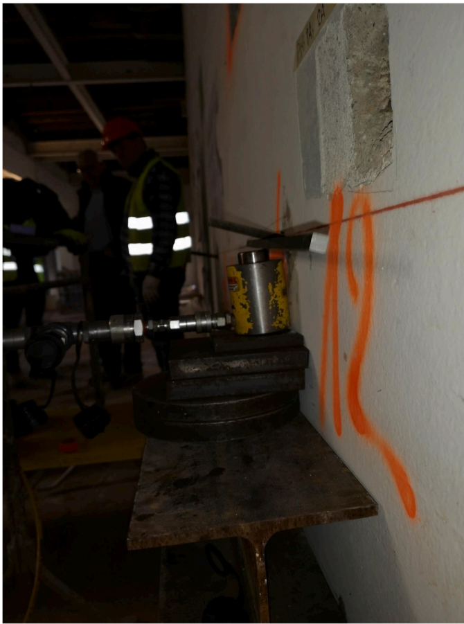
Fig. 9. Photo taken immediately after the test was completed. The image shows the anchor just tested, which is bent upward. This test used the square-section steel bar.
