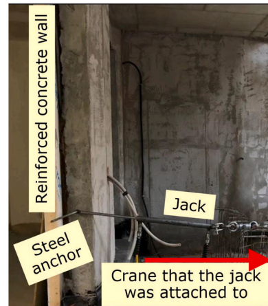
Fig. 11. This test used a set-up different than that described in Section 8. In this test, the force was applied by a jack that pulled the anchor and was restrained to a crane by means of a steel cable. This test was performed in the same building where a masonry shear anchor was tested as well [1], whose walls on the first story were made of concrete while on the upper stories were made of masonry.
