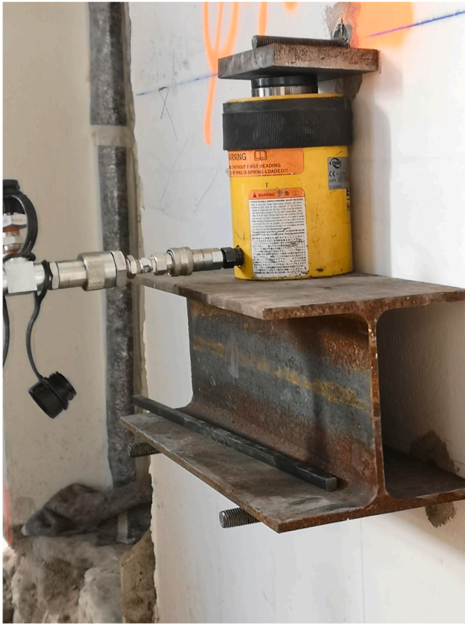
Fig. 7. Shear test performed using the procedure presented in Section 8. This test used a steel plate in lieu of the square-section steel bar because in so doing the eccentricity was lower (that bar appears on the I-section, unused).
