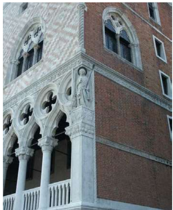
Fig. 2. Venice, Palazzo Ducale: the ‘noble’ stone and the ‘humble’ brickwork, the two main material components of Venice's architecture (Source: Squassina, 2010)
