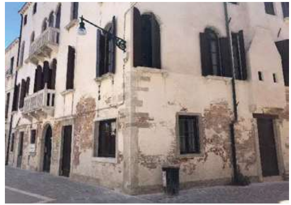
Fig. 5. New thick plasters cannot withstand the effect of rising damp for long in Venice: the above example is less than a decade old (Source: Squassina, 2021)
