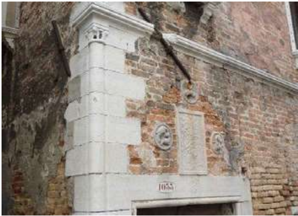
Fig. 3. Venice, Calle de le oche: detail of the gothic brickwork and a later cocciopesto plaster that have been bearing the effects of moisture and rising damp for centuries (Source: Squassina, 2012)
