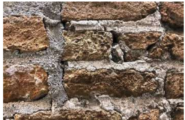
Fig. 4. Detail of medieval brickwork with well-polished lime-and-sand repointed joints (on the right) and a modern addition with a Portland cement mortar joint (left) highlighting the loss of traditional building skills (Source: Squassina, 2021)
