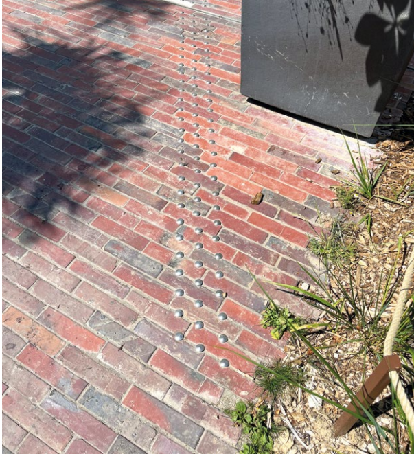
Fig.03 Incorrect placement of Tactile Indicators due the proximity to an obstacle.
