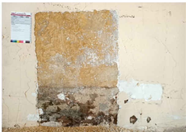
Fig. 7 Hall C, perimeter wall, sample No. 5: bichromy between the upper part, beige in color, and the brownish skirting ( Leonardo srl ).
