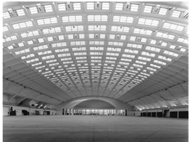
Fig. 3 Hall B, the appearance of the interior in white at present (courtesy of Fabio Oggero, 2022).
