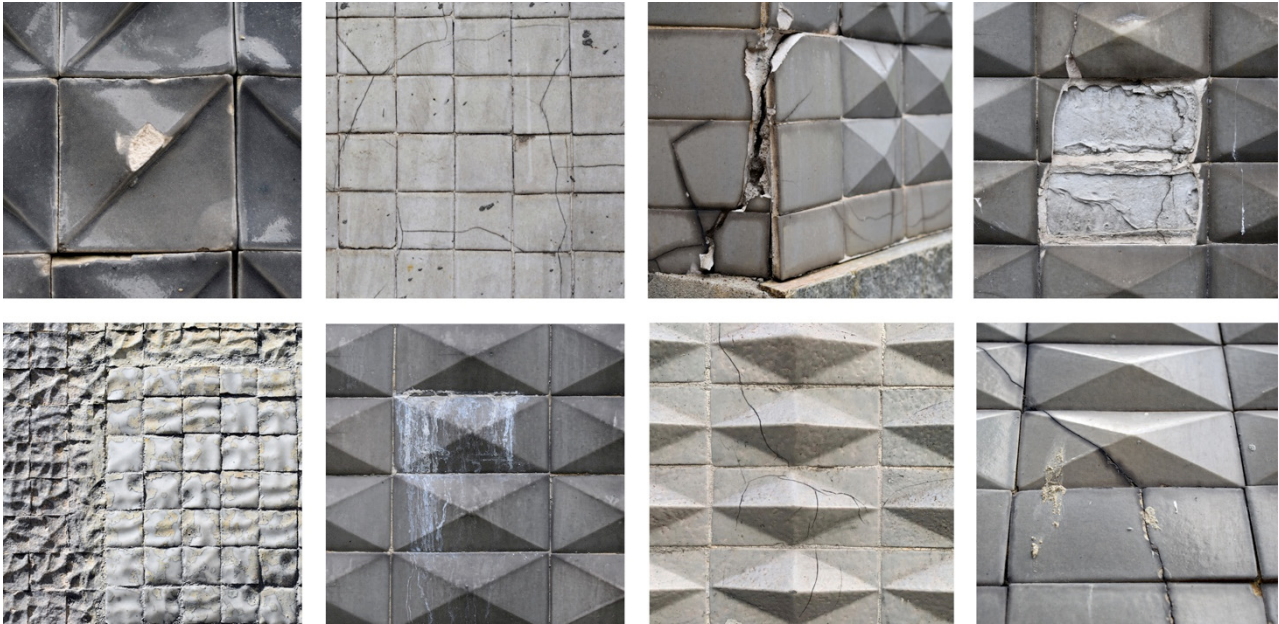
Fig. 7 Deterioration phenomena of modern ceramic surfaces. From top left: (a) expulsion of vitrification of glazed finishes; (b) hair cracks of unglazed porcelain tiles; (c) fractures of unglazed porcelain tiles due to the expulsion of concrete cover; (d) detachment and falling of mosaic tiles; (e) visually evident repair works; (f) deterioration of the cement mortar (substrate); (g) hair cracks on “diamond” unglazed porcelain tiles; (h) fractures on “diamond” unglazed porcelain tiles (Di Resta, 2021).
