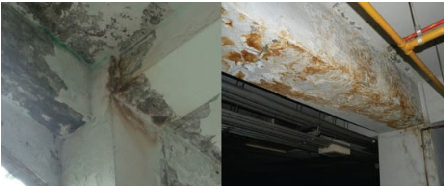
Fig. 1.2. Corroded beams in a RC building (From Ou et al. [50])
