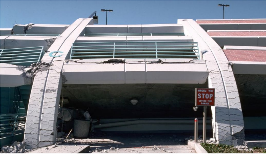
Fig. 1.1. Parking facility of California State University at Northridge (CA) partially collapsed during the 1994 Northridge Earthquake [23]
