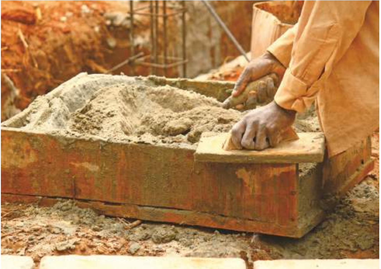
Moments of the building activity carried out by the students together with the local workers in the school complex in Zomai (Ouidah) during the internship trip to Benin in 2012.
