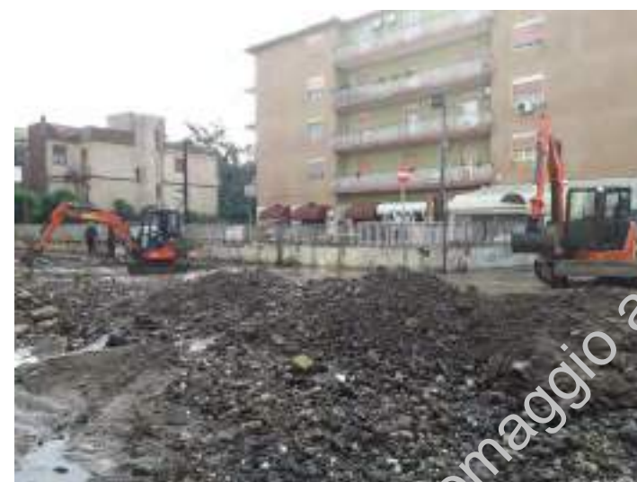
Fig. 2. Water bomb in the municipality of Scordia (CT) on 19 October 2018. (Source: Gaetano Giovanni Daniele Manuele).
