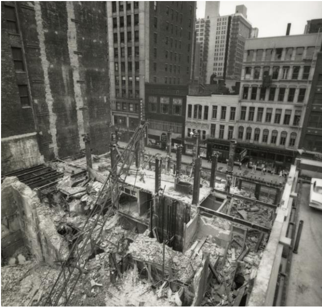
Fig. 5: Tower demolition, historical photograph (Richard Nickel, Burnham & Ryerson Library, The Art Institute of Chicago)
