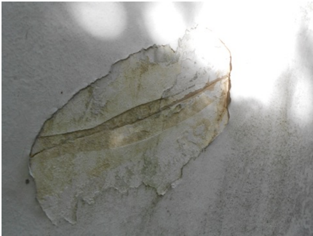
Figure 7. External surfaces decay, Eastern prospect, current state [Di Resta, 2015]
