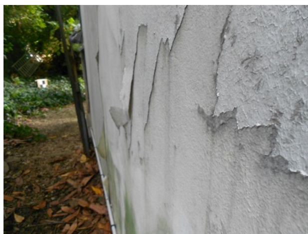
Figure 6. External surfaces decay, Eastern façade, current state [Di Resta, 2015]
