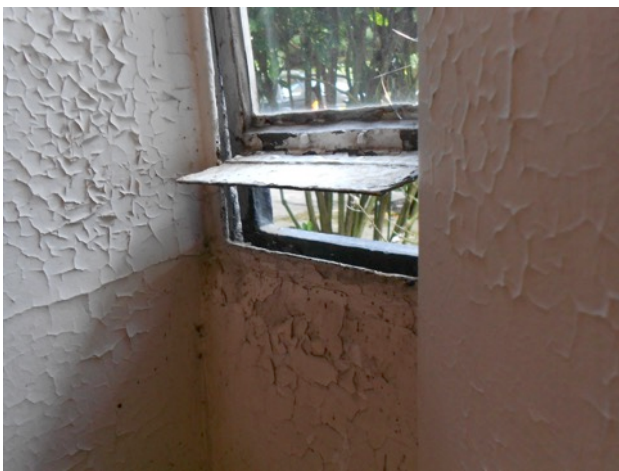
Figure 8. Internal surfaces and frames decay, current state [Di Resta, 2015]
