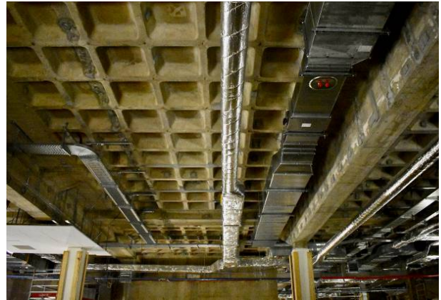
Fig. 6 Restoration site of the Neue Nationalgalerie, concrete structures of the basement with new pipes and the mock-up of false ceiling (Di Resta 2019).
