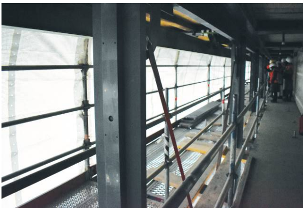
Fig. 5 Restoration site of the Neue Nationalgalerie, cross-bracing reinforcements to reduce deformation of steel components (Di Resta 2019).
