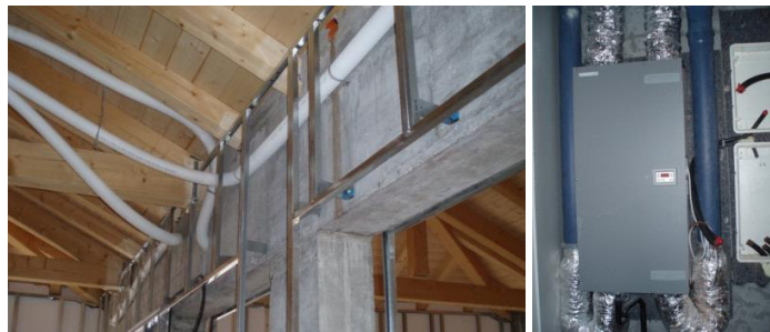
Fig. 5 Mechanical ventilation system.
