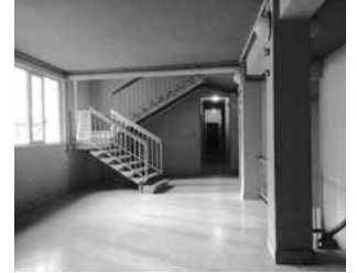
5F13 Interior view of the transitional space, showing the diagonal boundary of the staircase and the sloping soffit of the platform.
