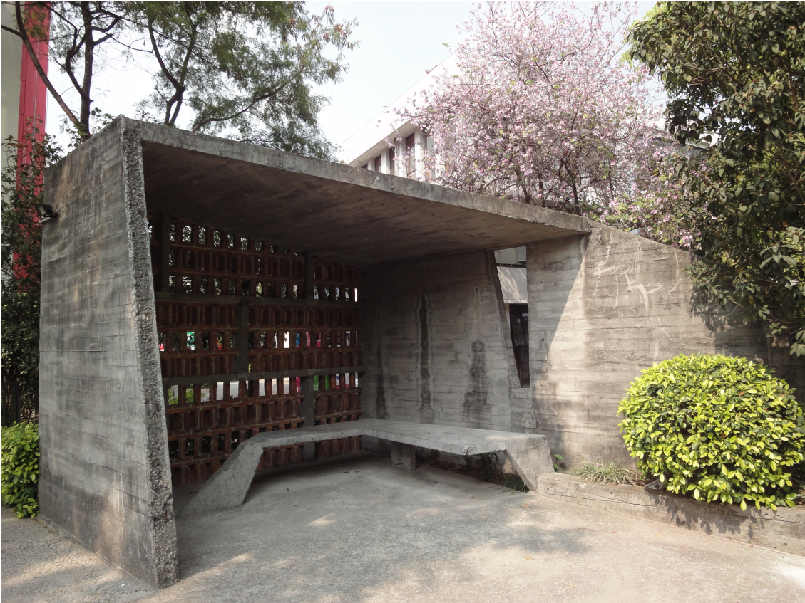
Figure 14. Detail of OCT Youth Hostel Renovation – point n. 9 in Figure 9 (on 27 th March 2012)
