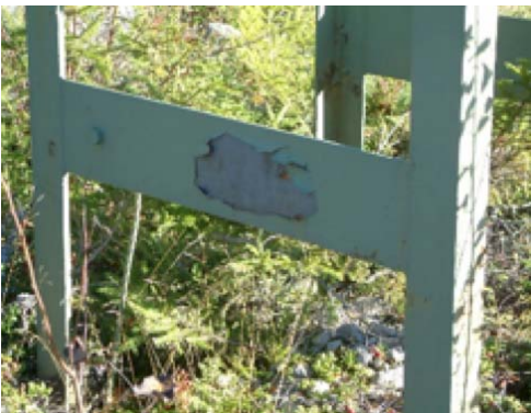
A 70-year-old coating starts flaking off
