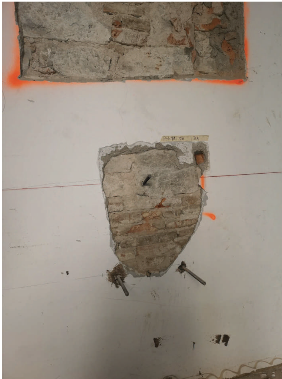
Fig. 11. Shear test performed in the case of a masonry made of bricks and stones, with lime mortar. The anchor was embedded into a stone of large size. The photo was taken after the test. The image shows the anchor just tested, which was bent upward, and the two lower anchors, which supported the steel beam and the jack. The upper part of the masonry (without plaster) had been tested in order to measure the mechanical characteristic of the masonry.
