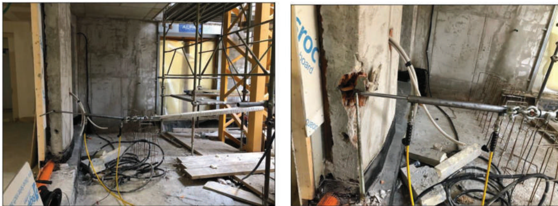
Fig. 13. Case study 5. This experiment was borderline, as it tested anchors post-installed into a masonry made of hollow bricks (perforated bricks, shown by the photo on the right), which required each anchor be enveloped by a sock.
