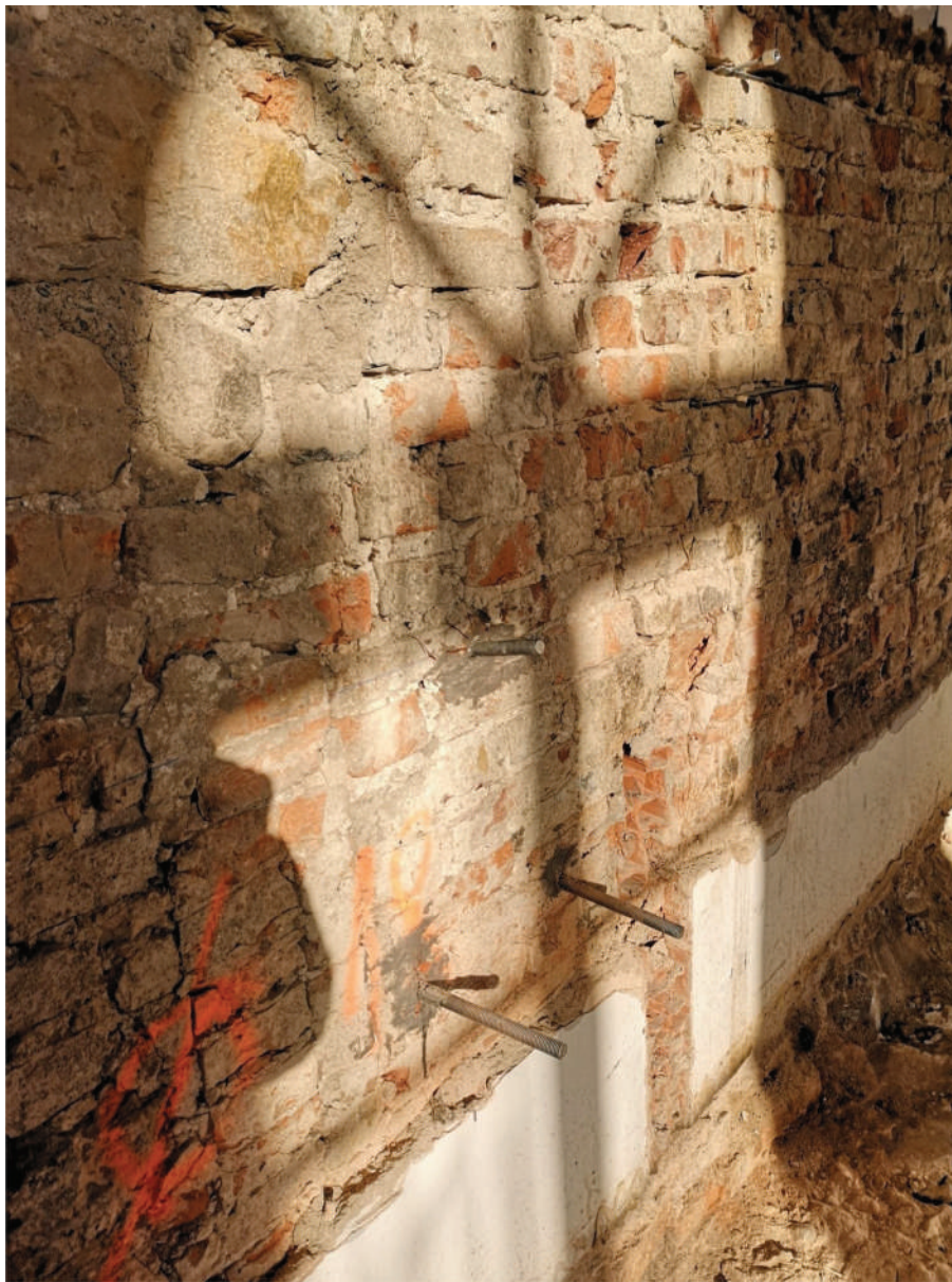
Fig. 8. Photo taken after having completed the test and having taken away the test set-up. The image shows the anchor just tested, which is bent upward, and the two lower anchors, which supported the steel beam and the jack during the test. On the top right the photo also shows the two flat jacks that had been used to measure the compressive strength of the masonry.
