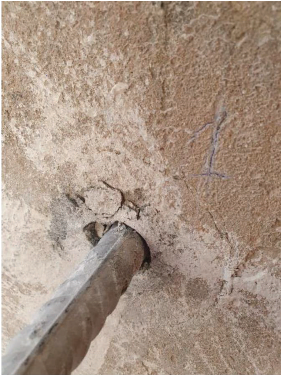
Fig. 12. Case study 4. Anchors after having reached collapse. This anchor was a rebar of diameter 200 mm. In this test the plaster could not be removed because of its high cultural and artistic value.
