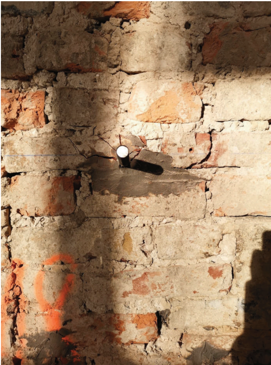
Fig. 10. Typical crack pattern at collapse. In every test when the anchor reached the maximum shear force that it could bear (failure), a vertical crack triggered at the upper point of the circular boundary of the drilled hole. Each test was continued increasing the anchor's rotation (and slightly decreasing the force applied by the jack). When the rotation increased, that crack propagated vertically upwards into the masonry. Then, other cracks triggered, with initiation at the upper semi-circumference of the drilled hole and with radial upwards propagation. In all the tests, the behavior softened only after rotations significantly larger than that at the maximum force (i. e., at the peak of load).
