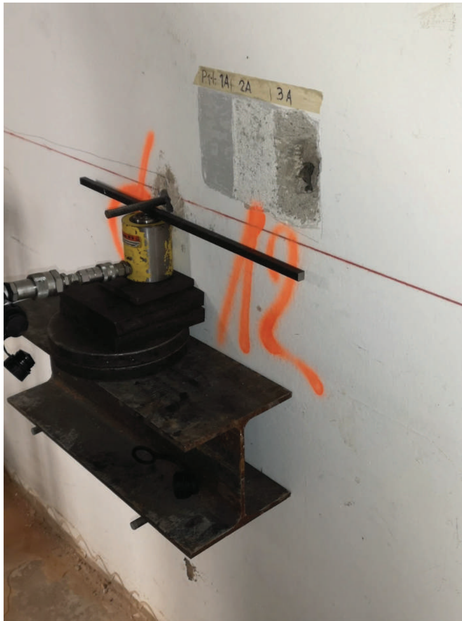
Fig. 7. Shear test performed on an anchor embedded into a masonry made of stones and lime mortar. In this test the plaster had not been removed because it consisted of a thin film. So, on one hand, the plaster did not alter the behavior of the anchor, while on the other hand, it allowed the cracks to be better observed and identified.
